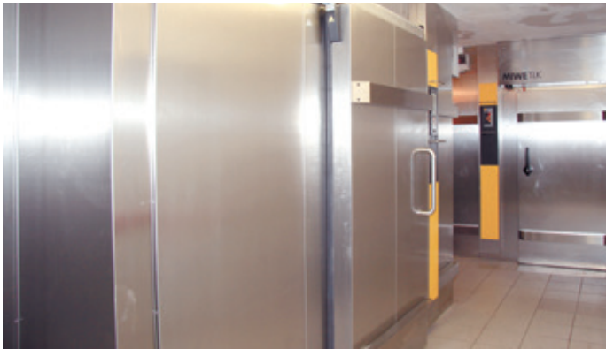
This modern bakery refrigeration system has been installed in the smallest of spaces – in the old barn.
