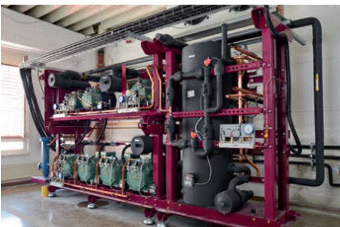
The technology for the refrigeration system is housed "neatly" in a separate room.
