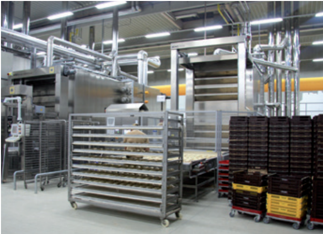
MIWE ideal M heating gas circulators are located beside the existing thermal-oil tunnel oven. Both were fitted with loading systems.
