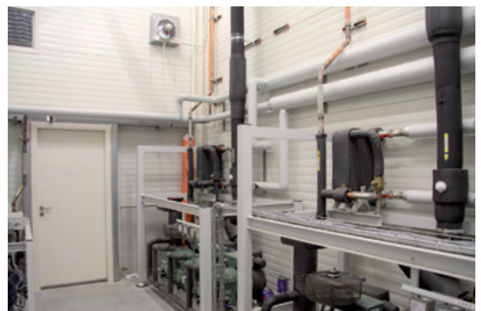
Plate heat exchangers recover heat from the refrigeration units and transfer it to buffer storage tanks for other uses.
