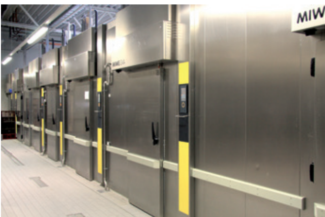
The freezer cabinets and fully automatic proofing block are installed as a compact system unit in the bakery.
