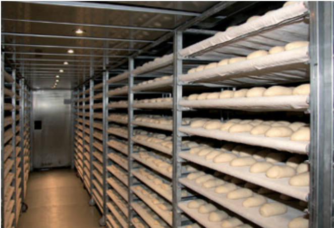
The combined systems in the bakehouse are especially fail-safe thanks to a second set of evaporators that is activated if the first one fails.
