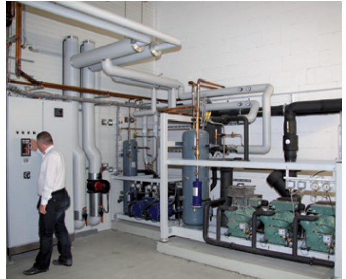
The refrigeration units are situated in a separate engineering room.
