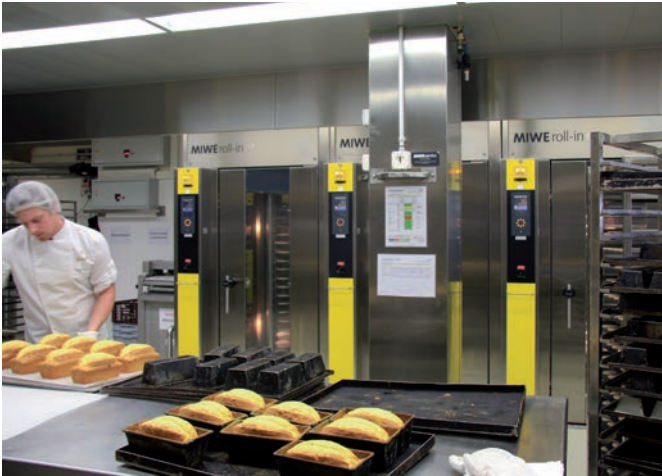
The roll-in e+ units were installed in one piece and integrated cleanly.
