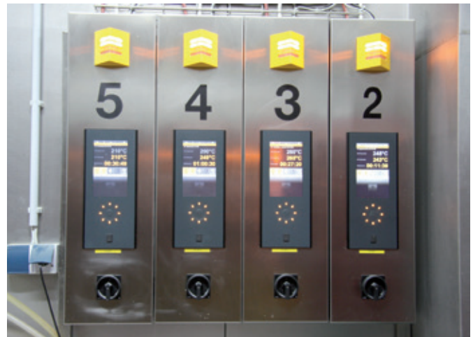
The MIWE thermo-static control system is in a separate location.
