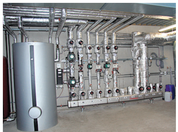
View of the technical room, which contains the buffer stores, among other things.
