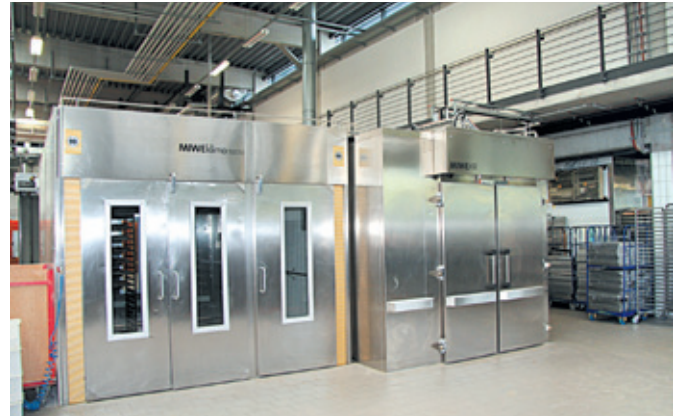
The bakery's baking and climate-controlled chambers.
