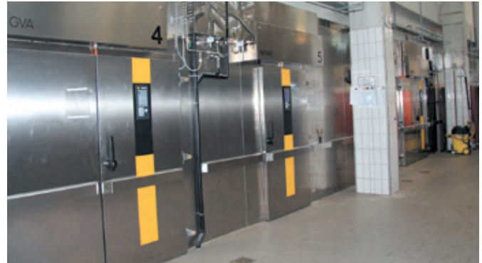
The bakery's cooling areas are located next to the production hall.
