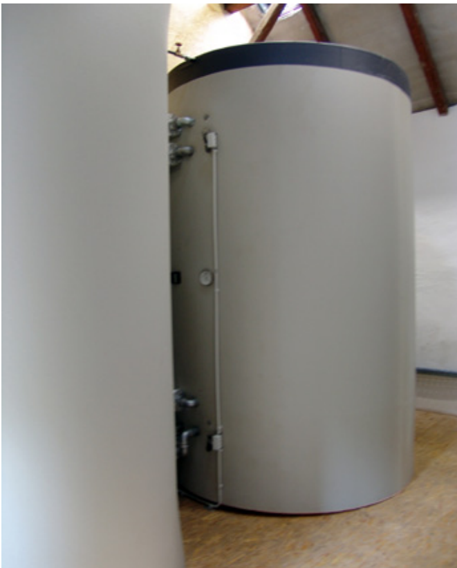
Two large buffer storage tanks, each of which can hold up to 13,000 litres of hot water, are situated on the former meal floor.
