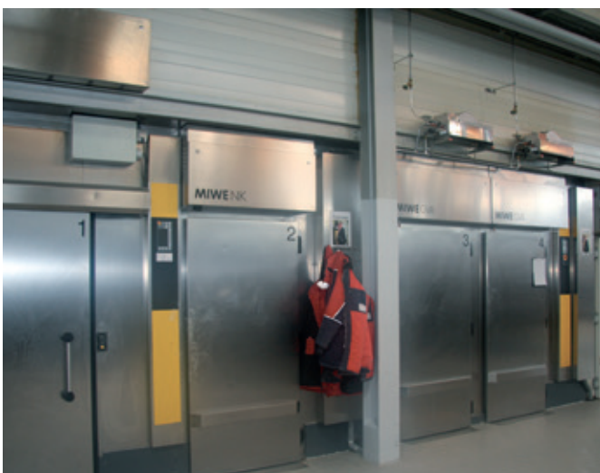
The refrigeration cells with flash freezers, normal refrigeration and fully automatic proofing units are attached to the side of the production hall.
