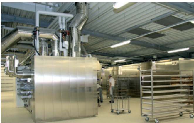
Only one exhaust flue to the roof is required since exhaust is routed from the baking ovens and the central boiler unit to the MIWE eco:nova.
