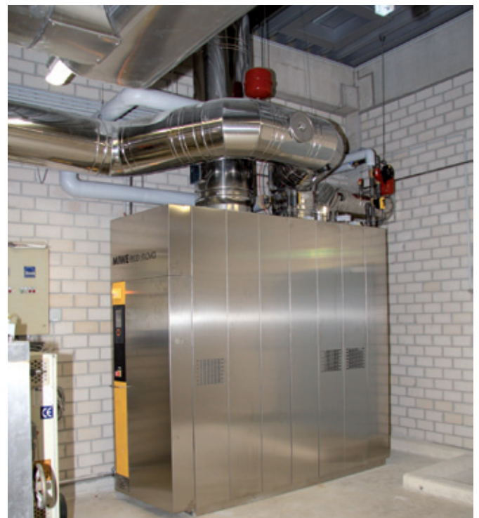
One MIWE eco:nova is supplied by flue gas from the central heating boiler for the thermal oil ovens. It is located directly beside the central heating boiler.
