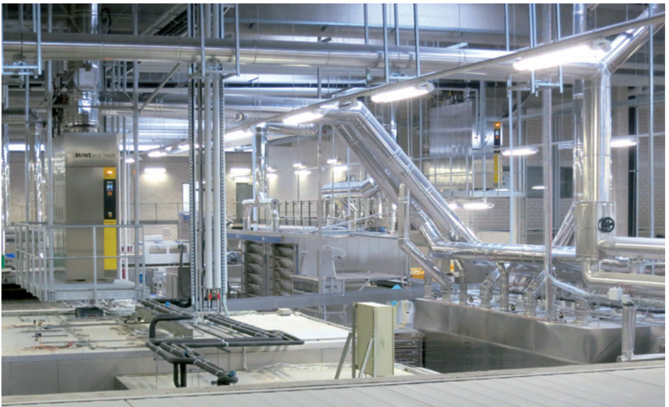
The excess energy from rack and wagon ovens is fed to a MIWE eco:nova which is installed via a cooling cell. This makes long pipelines unnecessary and saves space.
