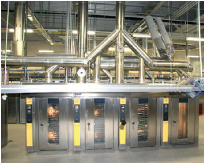
Flue gas and steam are routed separately from the rack ovens MIWE roll-in e+ (pictured) to a MIWE eco:nova. They receive further energy from the leftover steam from three thermal oil wagon ovens.
