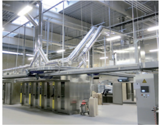
Surplus energy from the rack ovens in the form of hot flue gas and energy-rich steam can be made available for heat recovery.
