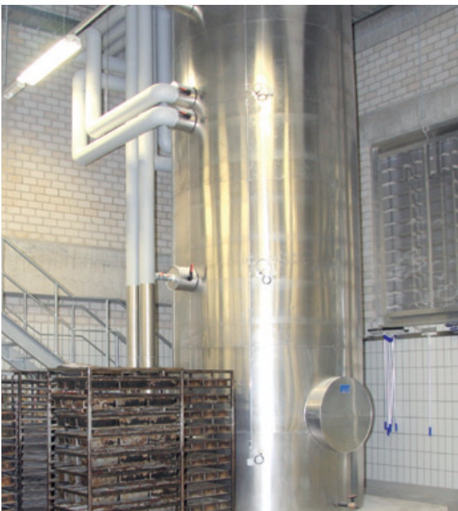
The multi-layer buffer storage tank has a capacity of 30,000 litres to store the recovered energy and provide it when required.
