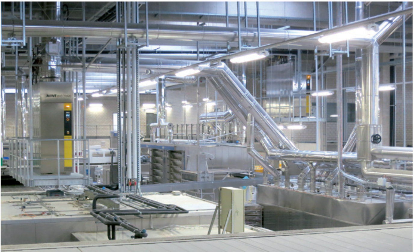
The excess energy from rack and wagon ovens is fed to a MIWE eco:nova which is installed via a cooling cell. This makes long pipelines unnecessary and saves space.
