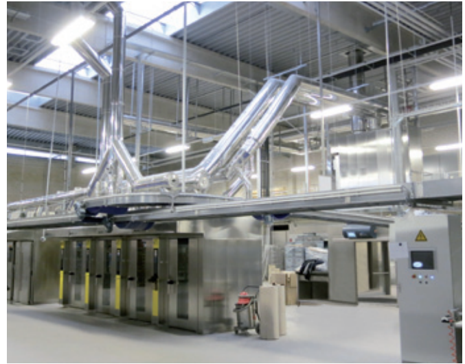
Surplus energy from the rack ovens in the form of hot flue gas and energy-rich steam can be made available for heat recovery.
