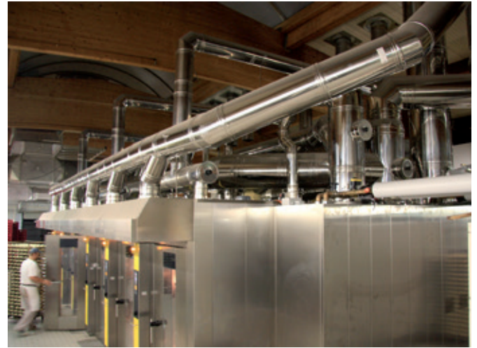
Flue gas and steam from the rack ovens on one side and from the MIWE ideal units on the other side are routed to the MIWE eco:nova heat recovery system (foreground). From there, just one chimney leads to the roof.
