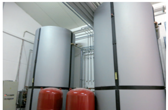
The MIWE eco : nova feeds the recovered energy to the buffer storage tank. From there, it is fed into the building services equipment.
