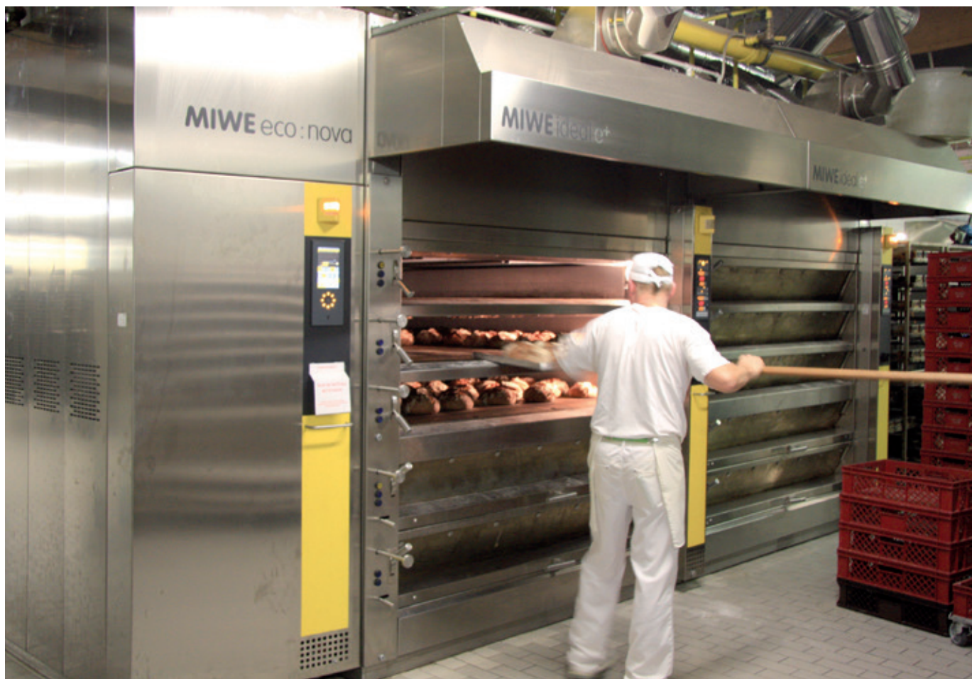
Two MIWE ideal e+ units are used primarily for bread. Right next to them is the MIWE eco:nova, which is also fed from the waste heat from central heating boiler.
