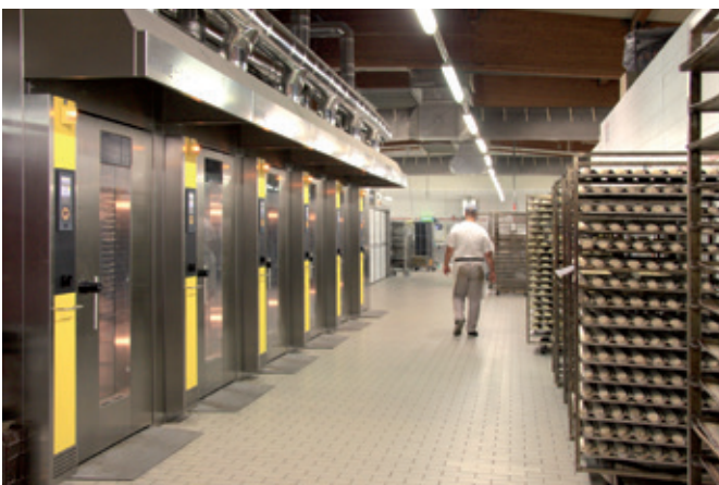
Thanks to 3D planning, MIWE was able to replace the ovens and commission the new energy saving units in record time
