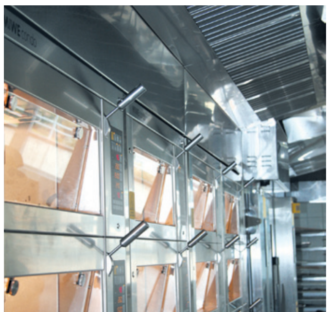
A generously dimensioned air duct positioned above the ovens ensures for a favourable climate in the apprentice bakeries.
