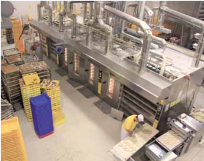
View of the ovens: wagon oven (centre) and deck baking ovens (left and right).
