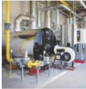
Central heating boiler: the core of the entire baking oven system
