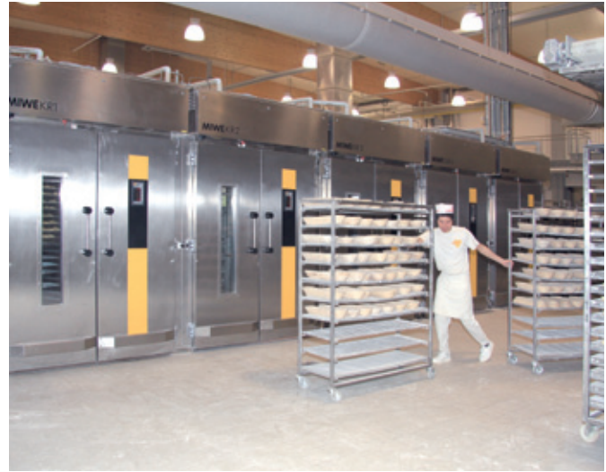
View of the bakery's climate and proofing chambers.
