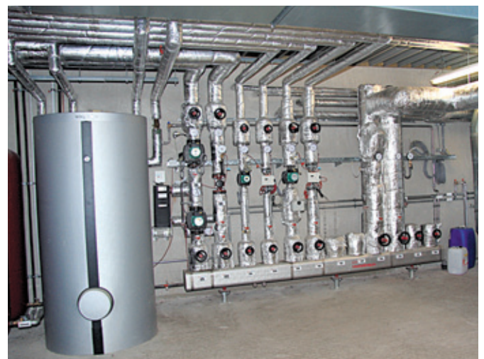
View of the technical room, which contains the buffer stores, among other things.
