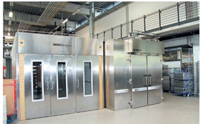
The bakery's baking and climate-controlled chambers.
