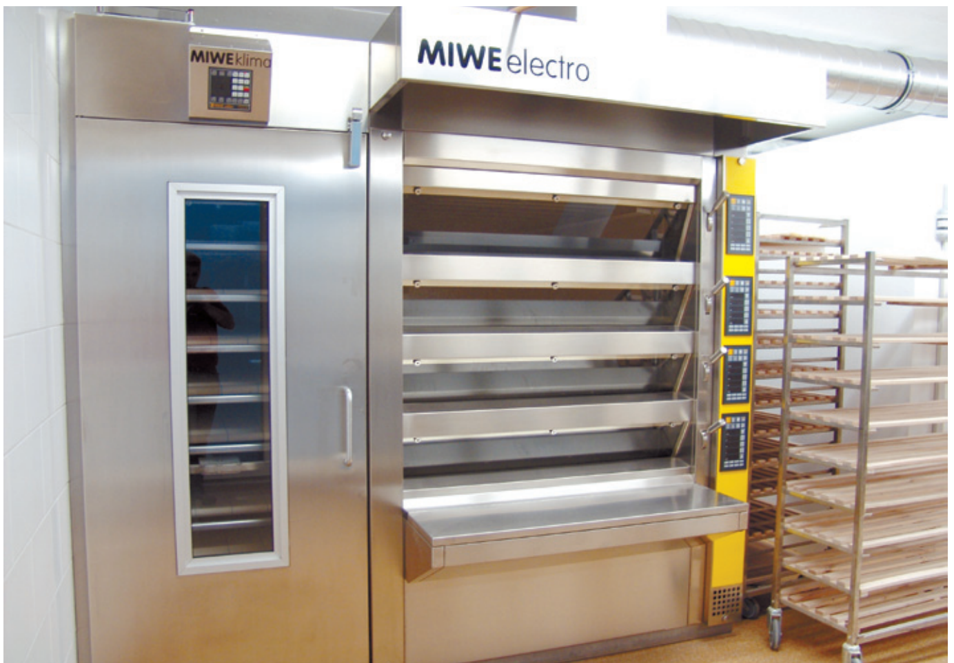
Front of the oven in the emergency bakery.
