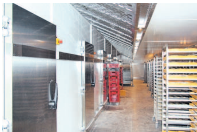
The refrigeration surface is amply dimensioned at Gellertstadt Backwaren. From the storage cells, the doors (left) lead straight to the fully automatic proofing units or from the freezing cells directly to the storage cells.
